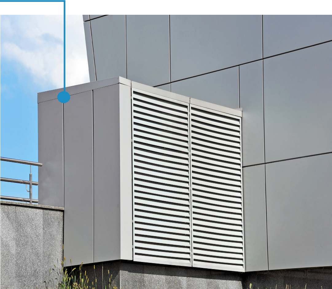
Industrial air conditioning and ventilation system at a hospital
