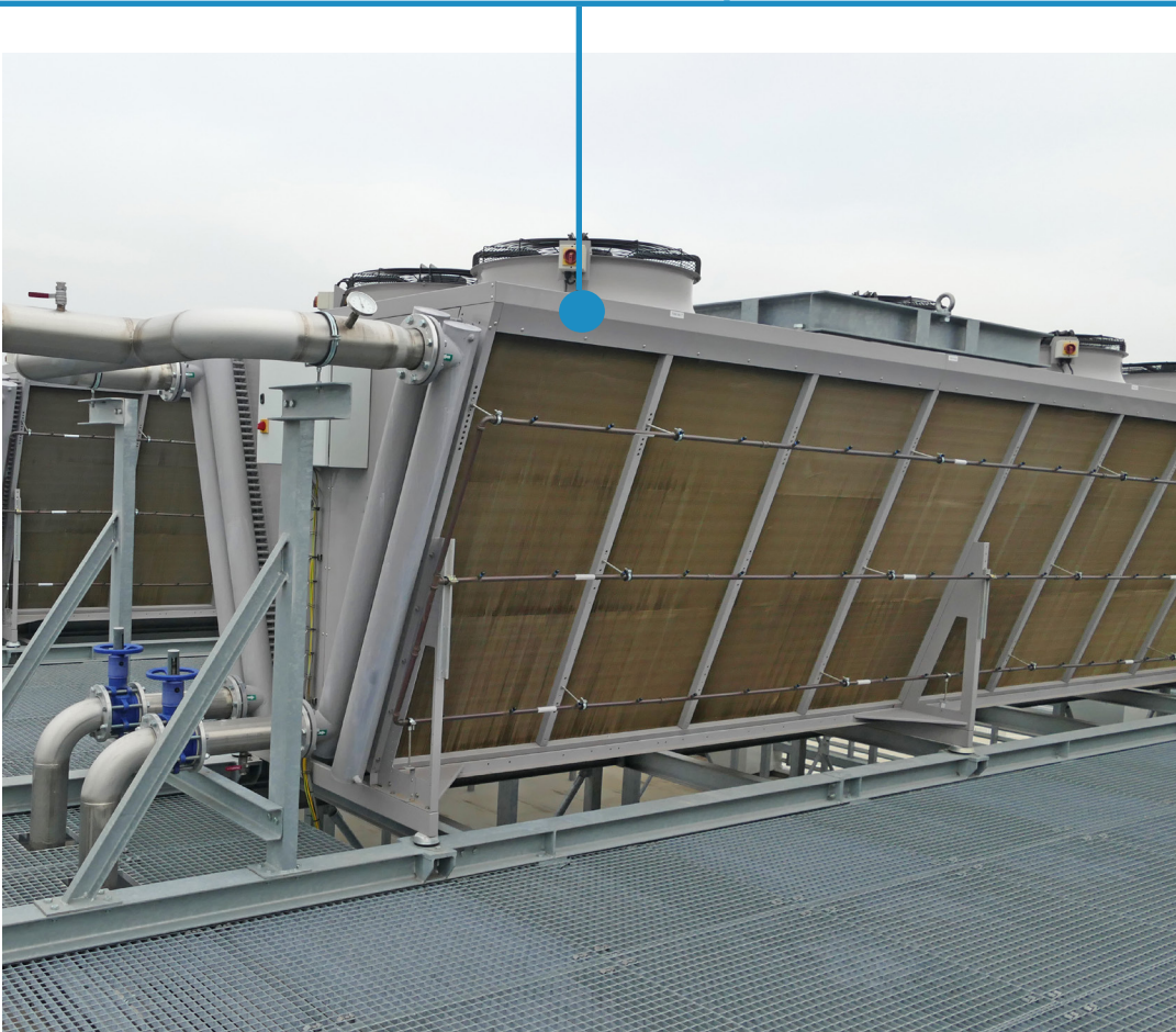
Chillers with fans cooling hot refrigerant on roof used in food industry manufacturing plant
